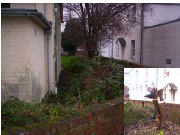
Before, and work in progress, at Christ Church Hall - part of the 'Clear Up Gloucester' campaign
